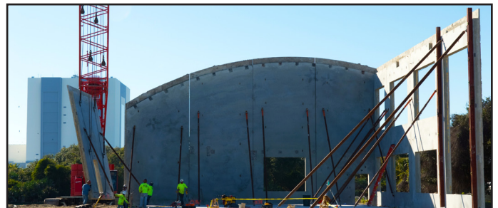
The walls of Propellants North are made of a THERMOMASS concrete wall insulation system. In this approach, the exterior layer of concrete is poured and leveled on the building's footprint. Then, prefabricated, predrilled insulation sheets are arranged on top of the un-hardened concrete, and connectors, designed to hold the sandwiched layers of concrete and insulation secure, are inserted through the predrilled holes. Next, the structural wythe is poured. Once cured, these panels are lifted upright to form the building's envelope.
