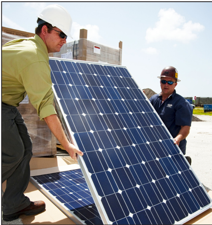
More than 300 solar panels were installed on the roof of Propellants North. Each panel will produce 235 watts of clean energy.
